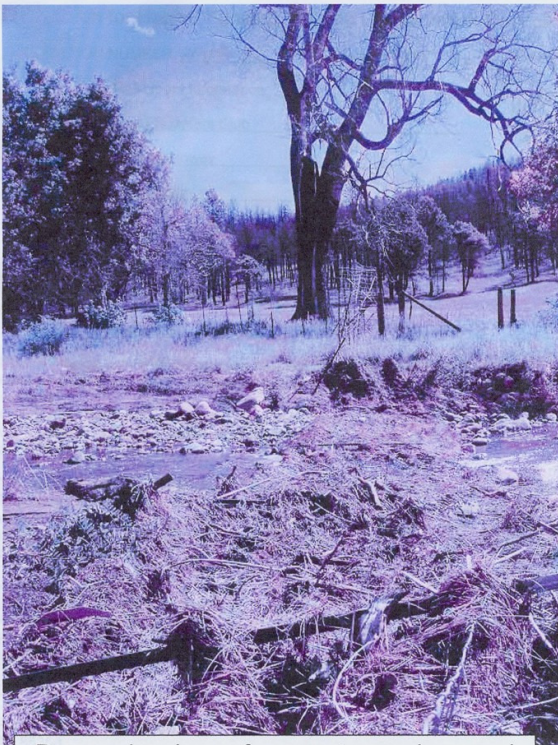
Damaged exclosure fence- water gap lower end Canyon Creek below OW Bridge
